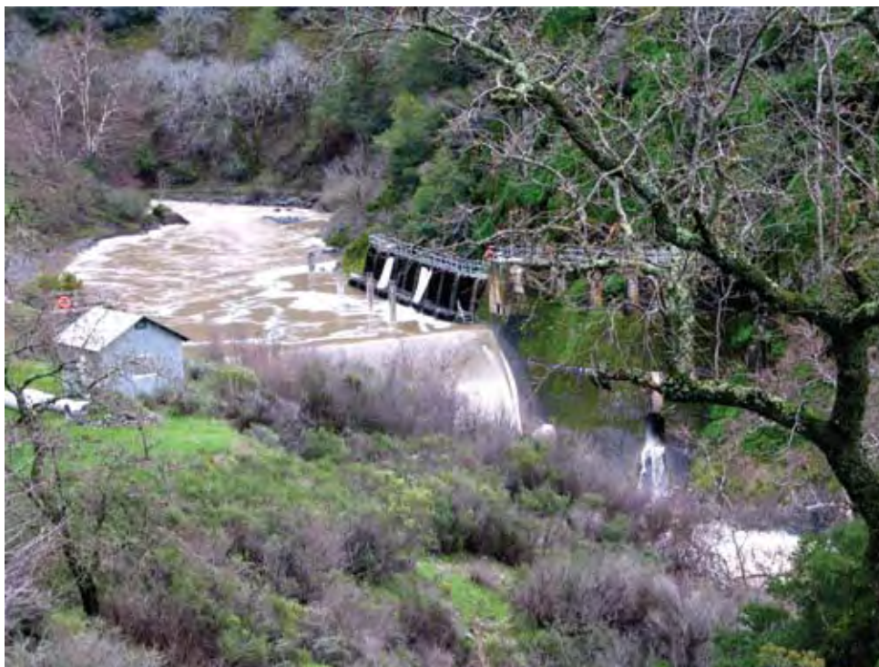
Alameda Creek Diversion Dam (a) during the dry season, and (b) during high flows sufficient to spill over the dam crest.
